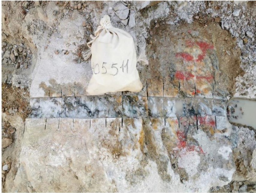
Fig 9.5. A channel cut over the quartz vein. Handy angle grinder is used.
